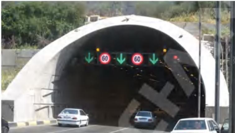
Installation Site: Iran
