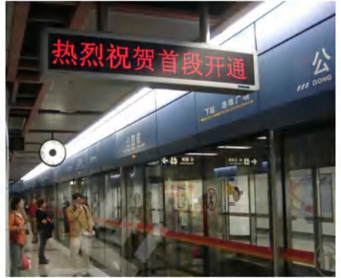
Installation Site: GuangZhou
