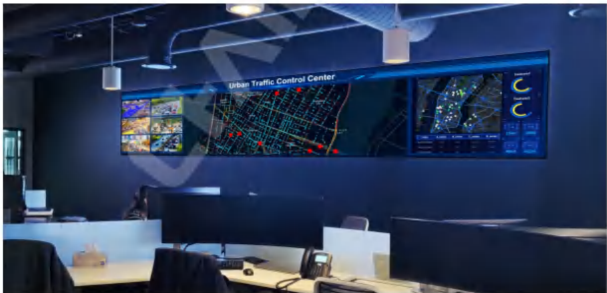
Installation Site: America
