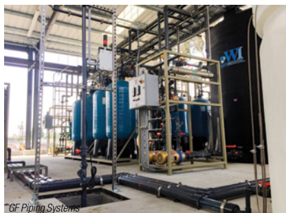
FIGURE 1. Water Innovations' HFX75d recycling system, supported by process-automation technologies from GF Piping Systems, reduced wastewater management costs for an aerospace manufacturer by 80%
