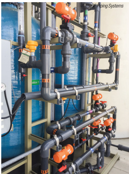
FIGURE 2. Specification of the proper components — from pH sensors to pressure-reducing valves — was critical to ensuring the success of the water-recycling system
