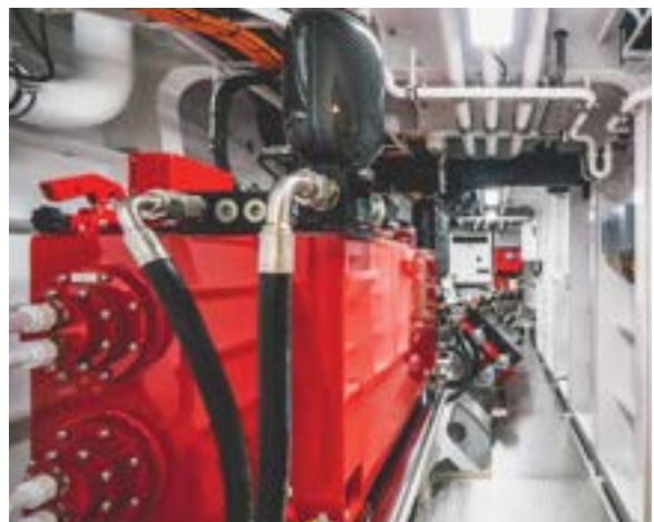
Stabilizer Room – 73m Feadship
