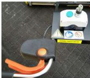
Main valve control
