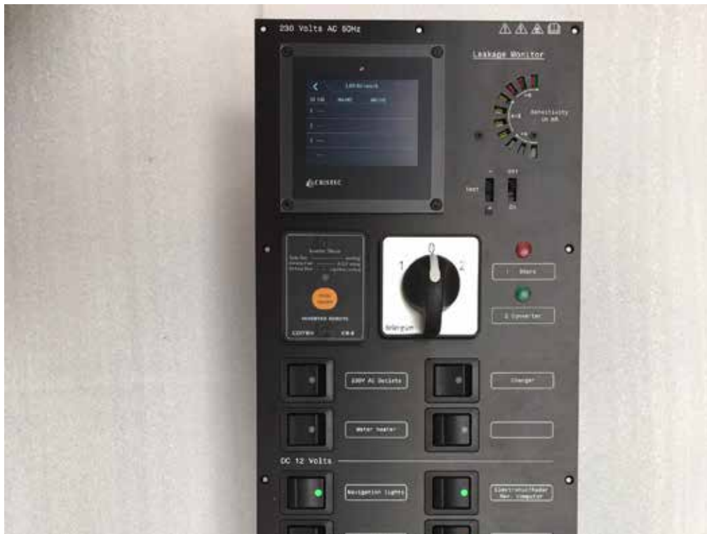
Example of BAT-MON monitor integration on a DC switching panel.
