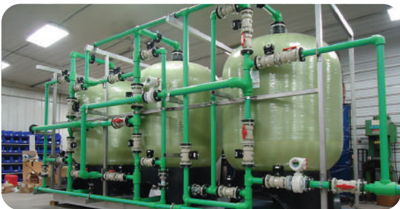
Industrial Water Treatment
