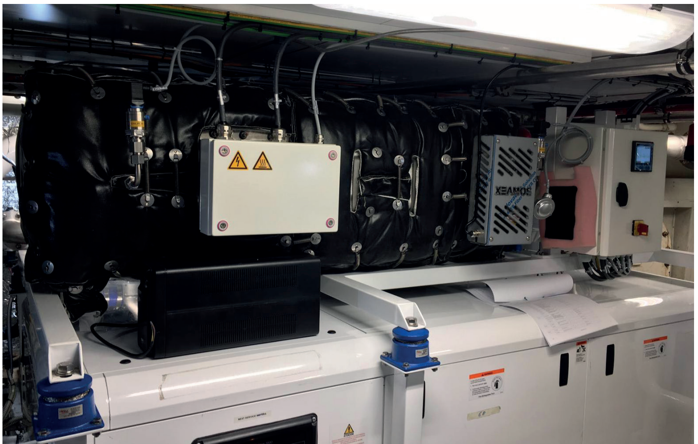
Example of installed DPF in existing engine room.
