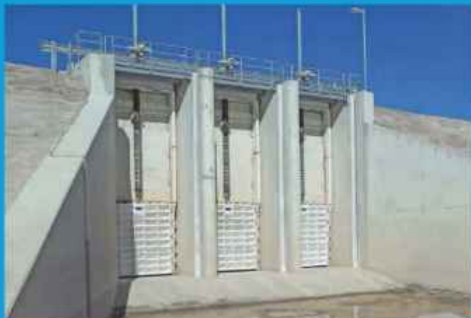
10' x 10', Cast Iron Slide Gates, Phoenix, AZ
